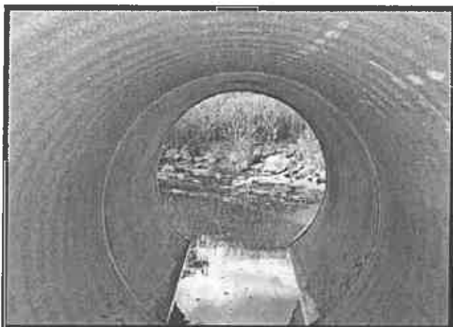
Drainage outfall used as a checkpoint for detection of illicit discharges in Pitt County.
