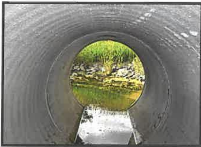
Drainage outfall used as a checkpoint for detection of illicit discharges in Pitt County.
